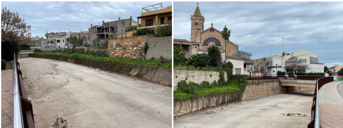
Figure 37. Flood canal and area affected most in 2018 in Son Carrió (Photos: Fekete, 25 Feb. 2025).
