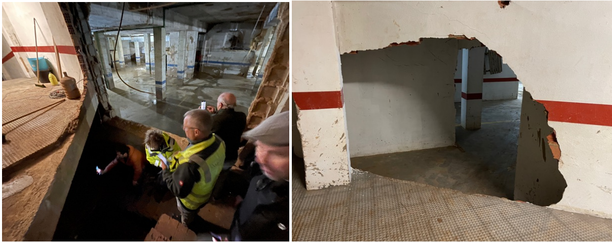
Fig. 7 Destroyed 3-storey underground parking garages in Catarroja (Fekete, 9.1.2025)
