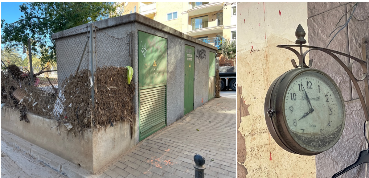
Fig. 10 Flood debris on the fence next to electricity infrastructure, stopped clock in a damaged café (Fekete, 9.1.2025)
