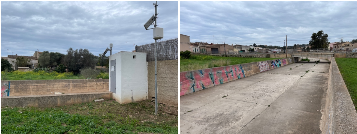
Figure 38. Flood canal in St. Llorenç and gauging and hydrometric station (Photos: Fekete, 25 Feb. 2025).
