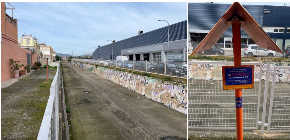
Figure 3. River canal of den Barberà crossing the Ma-13A, with concrete bed and walls, next to a car seller, and a warning sign of river level and exposed oil products in a flood, view to the north (Photos: Fekete, Palma, 25 Feb. 2025).
